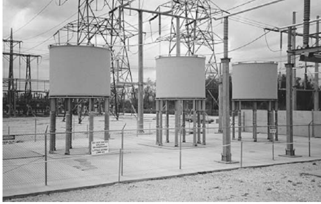
FIGURE 2.9.8 230-kV bus-tie reactors.
