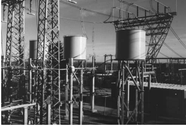
FIGURE 2.9.6 345-kV phase reactors.
