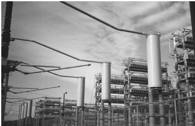
FIGURE 2.9.16 550-kV capacitor inrush/outrush reactors.
