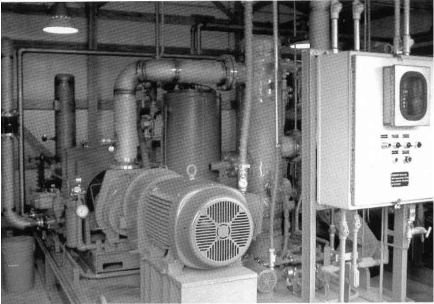
Figure 17-4. Gas Compression System
