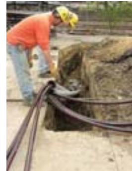
Underground transmission system.
